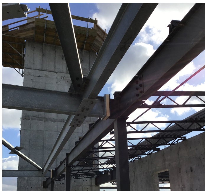
Different thermal breaks used in the Fire Hall No.17 envelope construction (Credit: HCMA)
