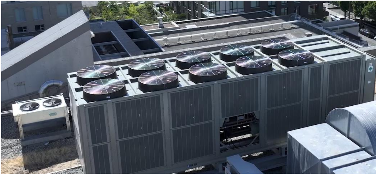
FIGURE 66: THE NEW ASHP AT THE ATRIUM
