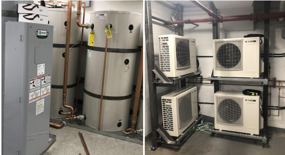
FIGURE 71: THE NEW DHW SYSTEM AT ARTHUR ERICKSON PLACE
